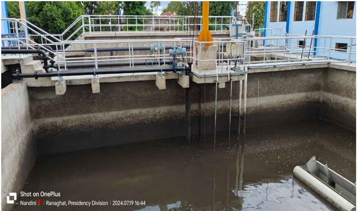
STP at Silver Jubilee Road - Ranaghat, Nadia
