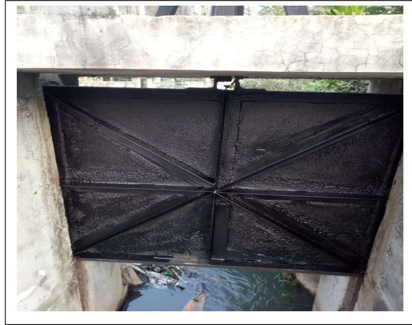
HALISAHAR DRAIN LOCKGATE
