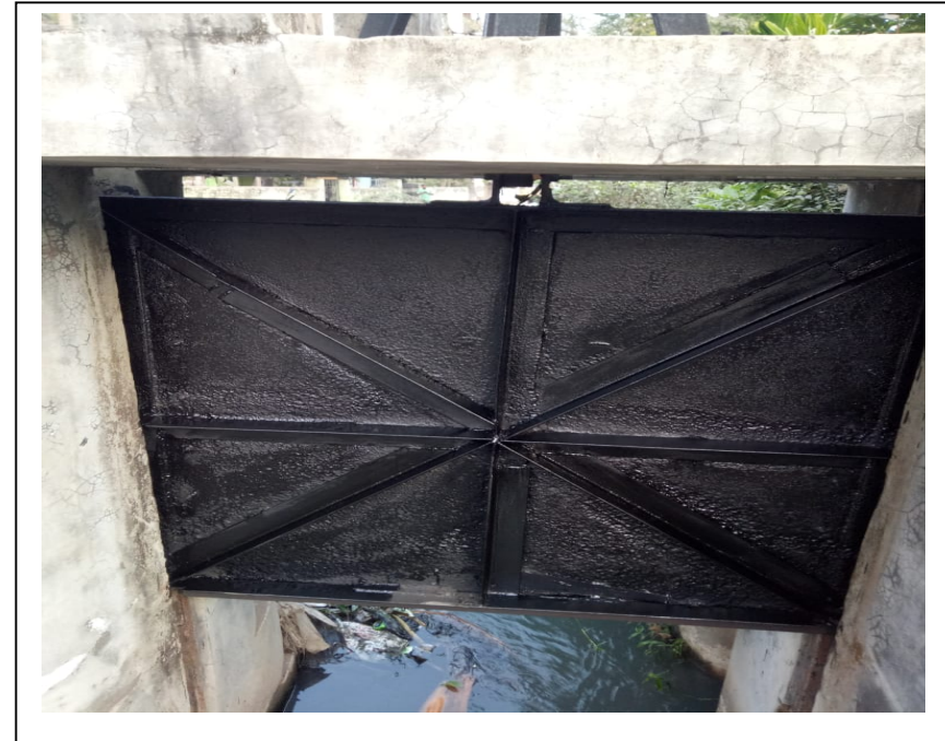
HALISAHAR DRAIN LOCKGATE
