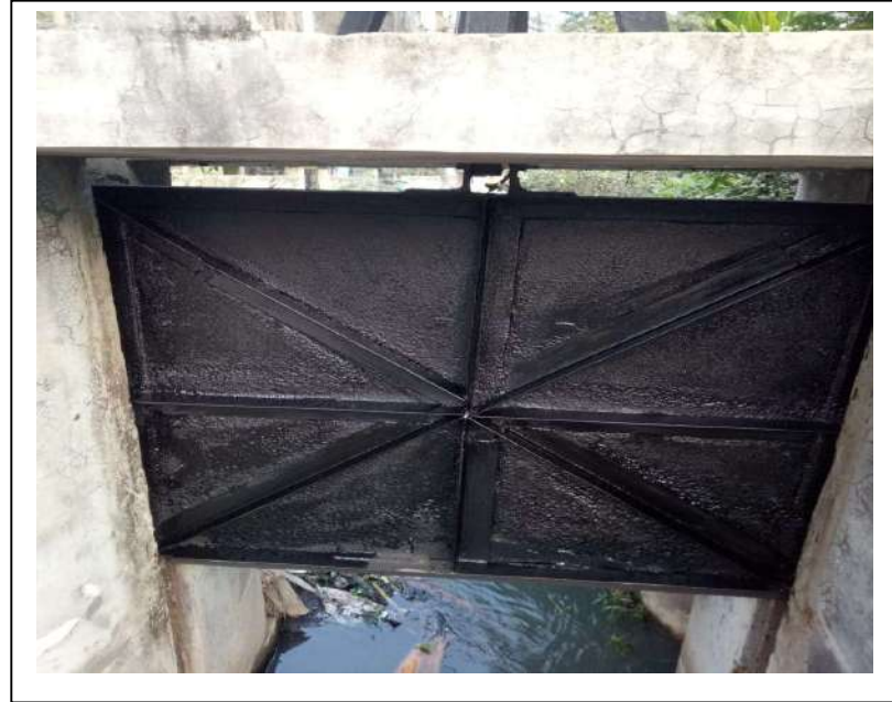
HALISAHAR DRAIN LOCKGATE
